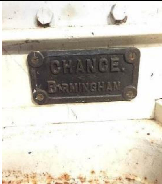
Figure 35. Maker plate in place on rotating machine: 'Chance. Birmingham'
